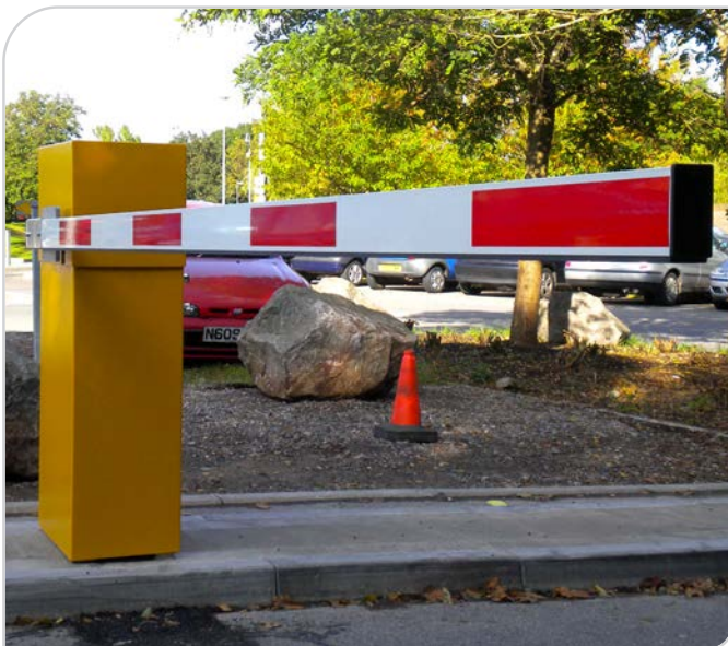
Installed automatic raising arm barrier
